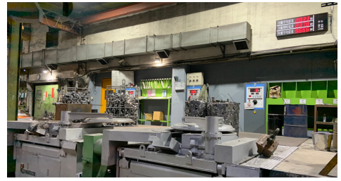
Introducing mid-frequency furnace decreases energy consumption by 8% during production, and create green casting achievement.
